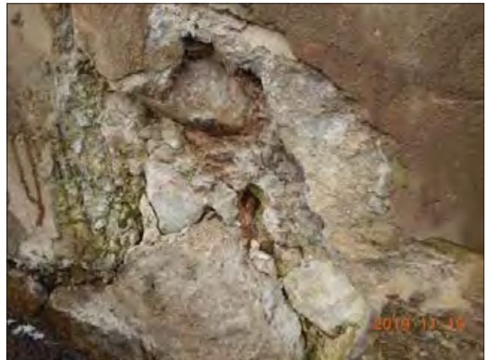
Photo 2767 - Sept 19, 2019 Pefferlaw Dam
