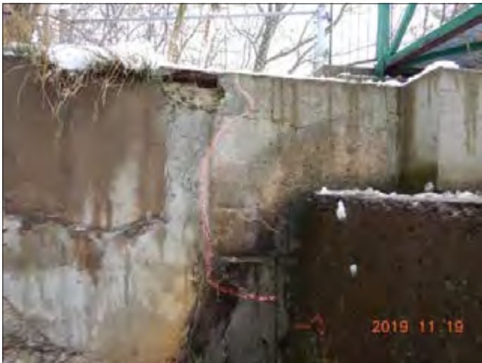
WILLS WATERSHED Lake Simcoe Region Conservation Authority Photo 2841 - Sept 19, 2019 Pefferlaw Dam Right (East) Dam Abutment
