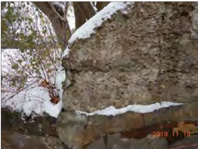
WILLS WATERSHED Lake Simcoe Region Conservation Authority Photo 2839 - Sept 19, 2019 Pefferlaw Dam Right (East) Dam Abutment
