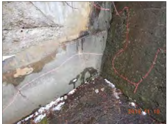
WILLS WATERSHED Lake Simcoe Region Conservation Authority Photo 2840 - Sept 19, 2019 Pefferlaw Dam Right (East) Dam Abutment
