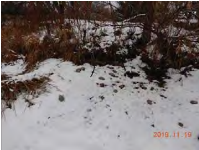
WILLS WILSON CONSULTANTS Lake Simcoe Region Conservation Authority Photo 2670 - Sept 19, 2019 Pefferlaw Dam Upstream Right Earth Embankment
