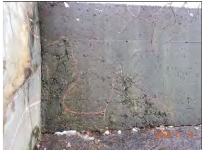
WILLS WATERSHED Lake Simcoe Region Conservation Authority Photo 2842 - Sept 19, 2019 Pefferlaw Dam Downstream Side of Right (East) Weir
