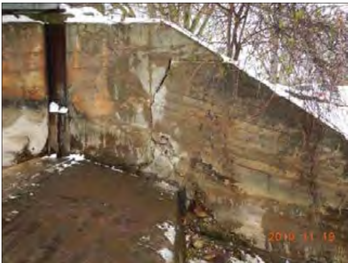
Photo 2764 - Sept 19, 2019 Pefferlaw Dam
