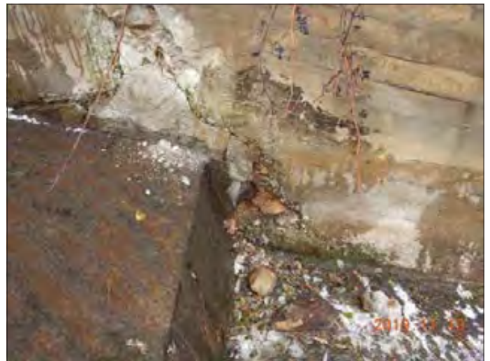
Photo 2765 - Sept 19, 2019 Pefferlaw Dam
