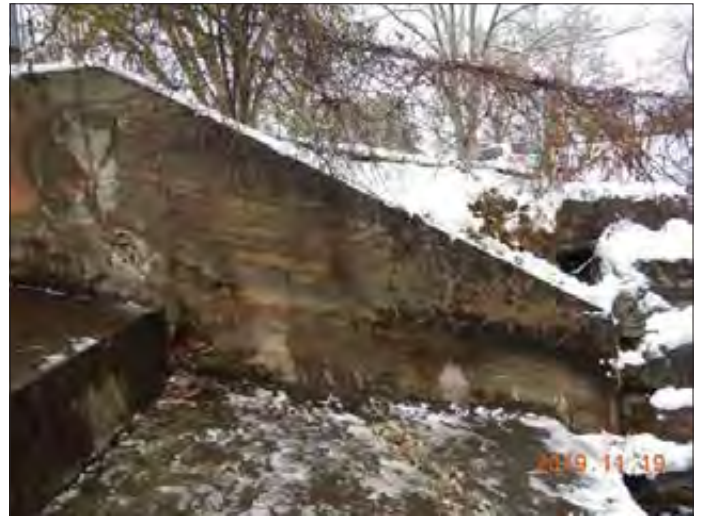
Photo 2763 - Sept 19, 2019 Pefferlaw Dam
