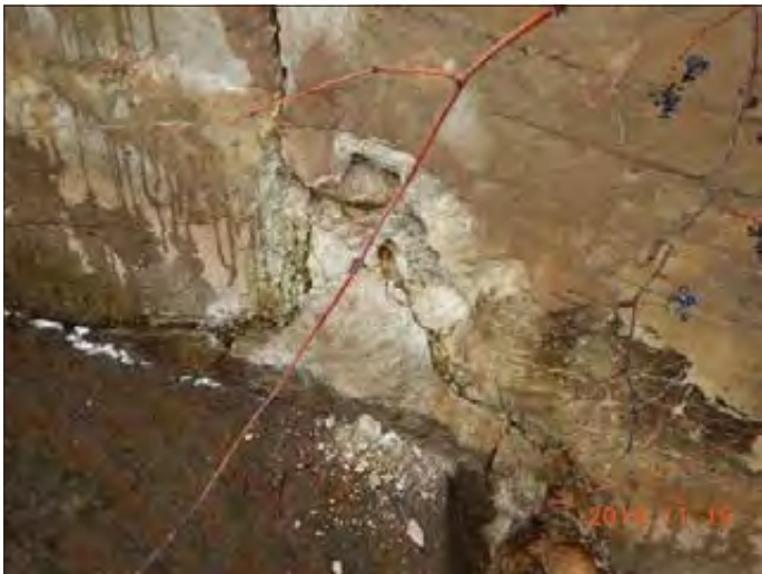
Photo 2766 - Sept 19, 2019 Pefferlaw Dam
