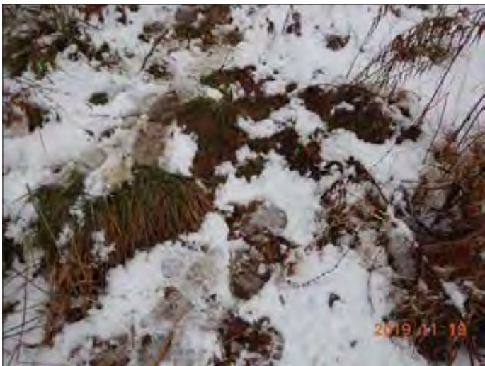
WILLS WILSON CONSULTANTS Lake Simcoe Region Conservation Authority Photo 2674 - Sept 19, 2019 Pefferlaw Dam Upstream Right Earth Embankment
