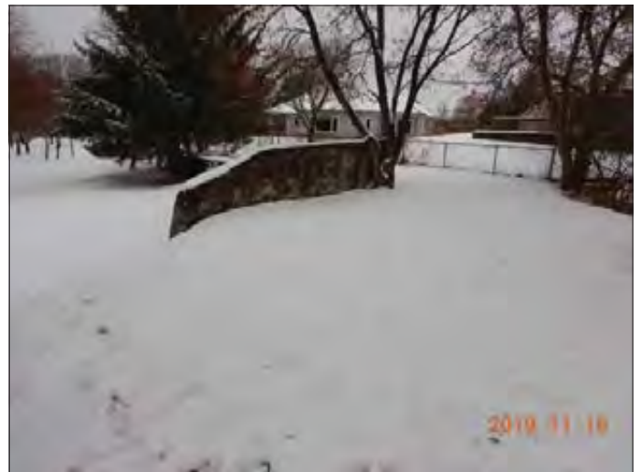
WILLS WILSON CONSULTANTS Lake Simcoe Region Conservation Authority Photo 2676 - Sept 19, 2019 Pefferlaw Dam Right Earth Embankment Crest
