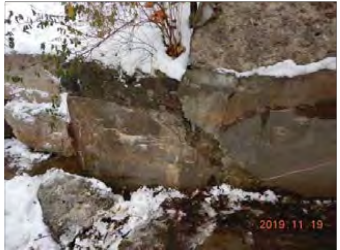
WILLS WATERSHED Lake Simcoe Region Conservation Authority Photo 2838 - Sept 19, 2019 Pefferlaw Dam Right (East) Dam Abutment
