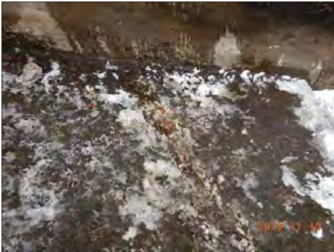
Photo 2762 - Sept 19, 2019 Pefferlaw Dam
