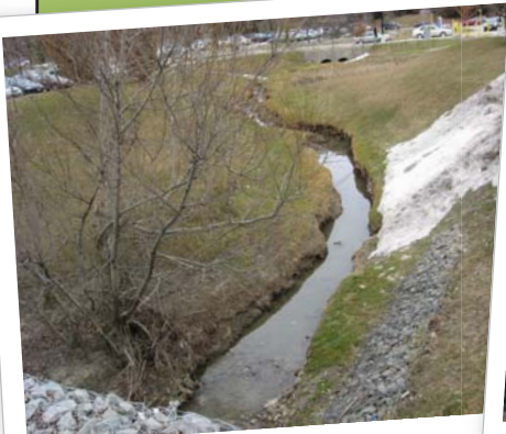
Streambank erosion: March 2007
