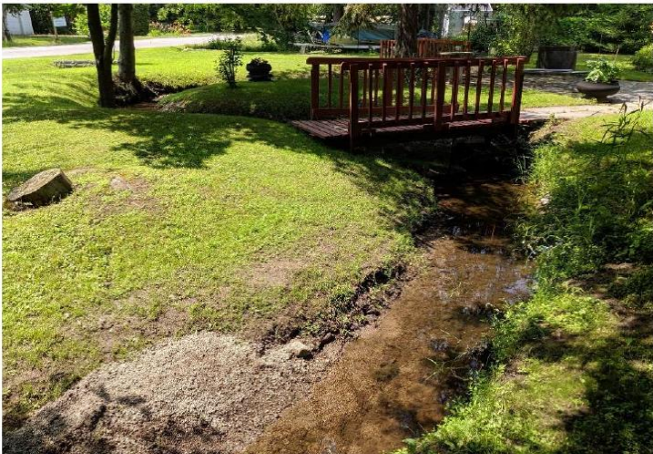
Figure A 1 Belle Aire creek near 1056 Spruce Road – limited conveyance capacity
