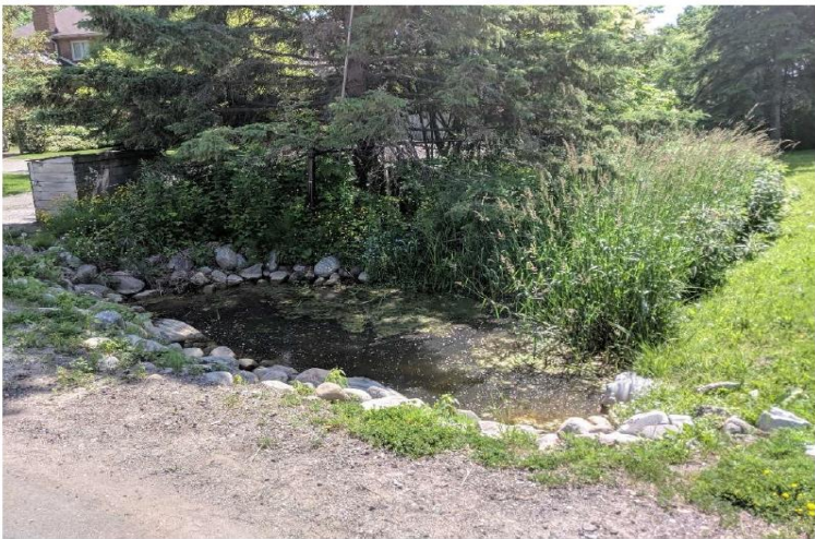
Figure A 3 Culverts along Belle Aire creek - Inadequate size
